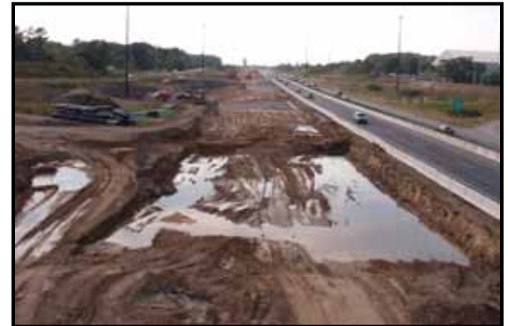
Looking West from Hwy 169 overpass during construction reveals the extraordinary high water table in this location
