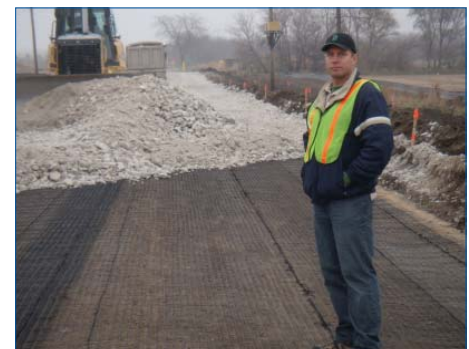
A representative from the local distributor is on site to offer support during installation.
