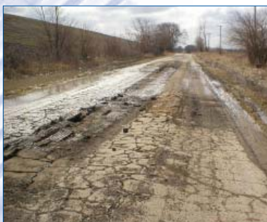
Much of Bungalow Road remained saturated due to overgrown ditches and poor soils; eventually leading to complete failure.
