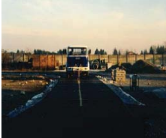
MS Multi-Layer Geogrids have been installed and tested for performance in comprehensive in-ground testing
